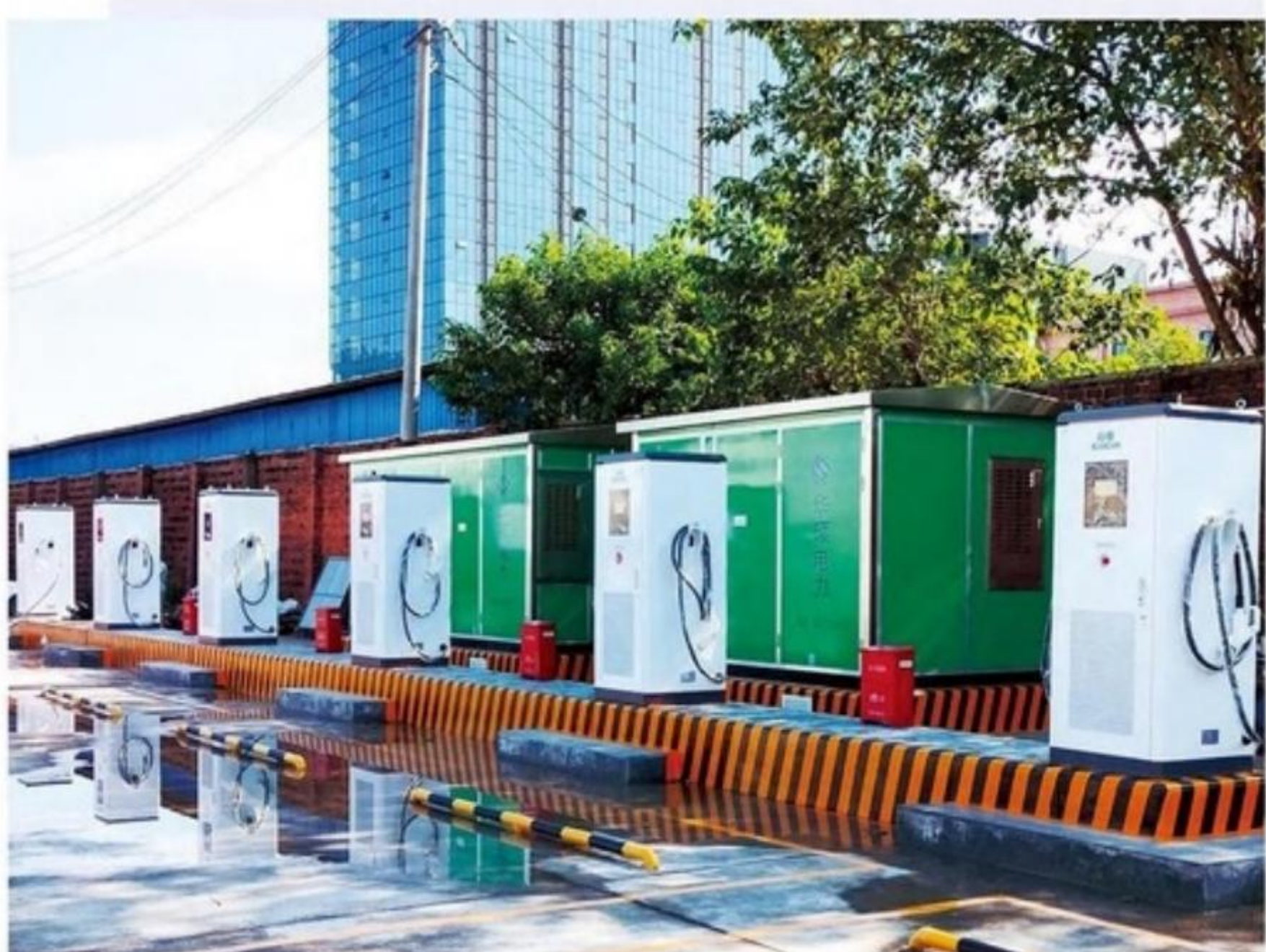
Guigang Green Card Charging Station in Guangxi
